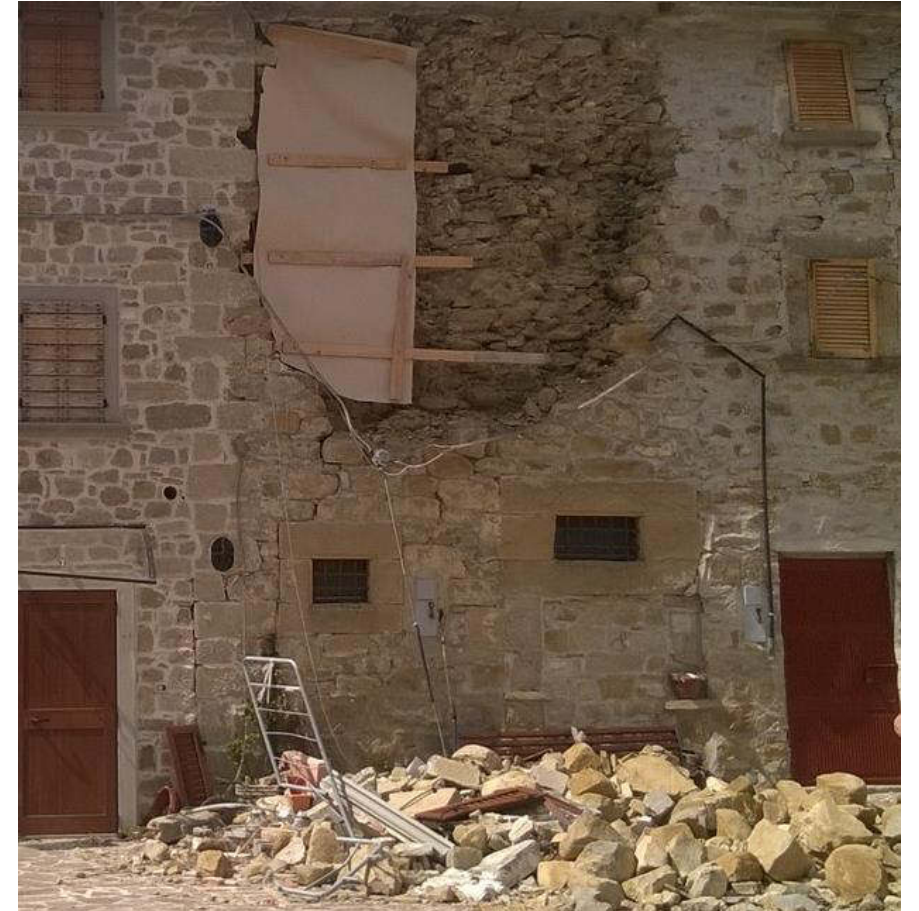
Montegallo, Frazione Colle
